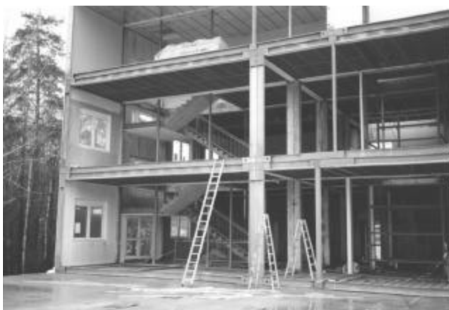
Fig. 1: Frame structure of the building radiation protection relevant data, a separate top floor which houses all equipment for air conditioning, ventilation and filtering). The building is constructed from prefabricated standard room containers. The dimension of such a container is 3.3 x 6.6 x 8.3 m (height x width x
