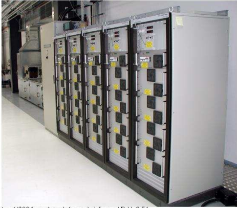
Status 1/2004: each rack (smps) delivers 15kV, 2.5A
